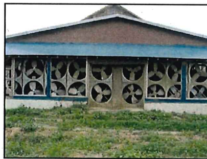
↑牛舎壁面の換気扇
